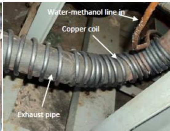
Fig. 4.12 Copper Coils to the Exhaust Pipe for the Production of Vaporized Water-Methanol.
