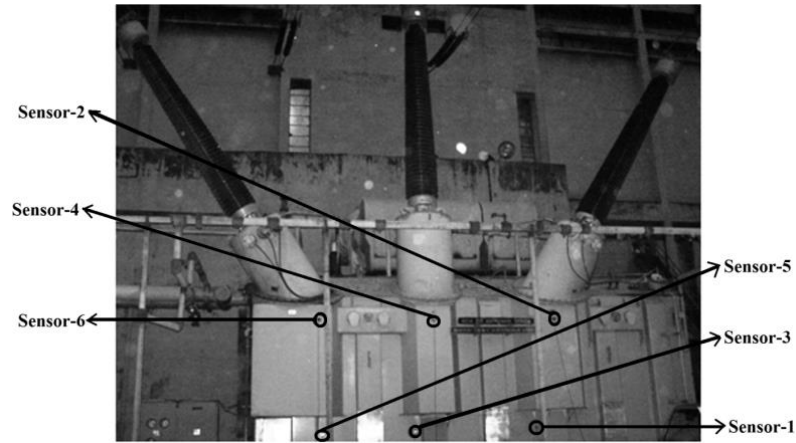
Figure 2.2: View of 250 MVA 15.75 kV/420 kV GT with sensors mounted (sensors mounted on the HV side of transformer tank are seen)
