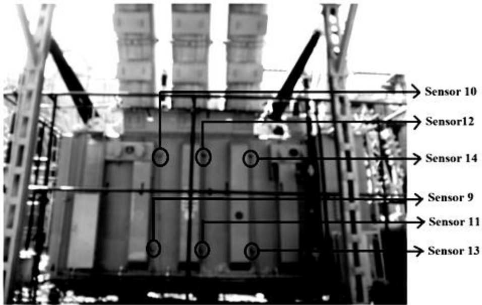
Figure 2.11: View of 123 MVA 13.8 kV/420 kV GT with sensors mounted (sensors mounted on the LV side of transformer tank are seen)
