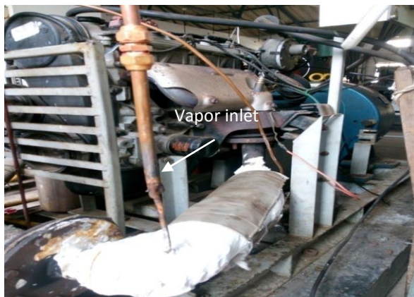
Plate 3.7 Heat exchanger for production of vapor of water-methanol.
