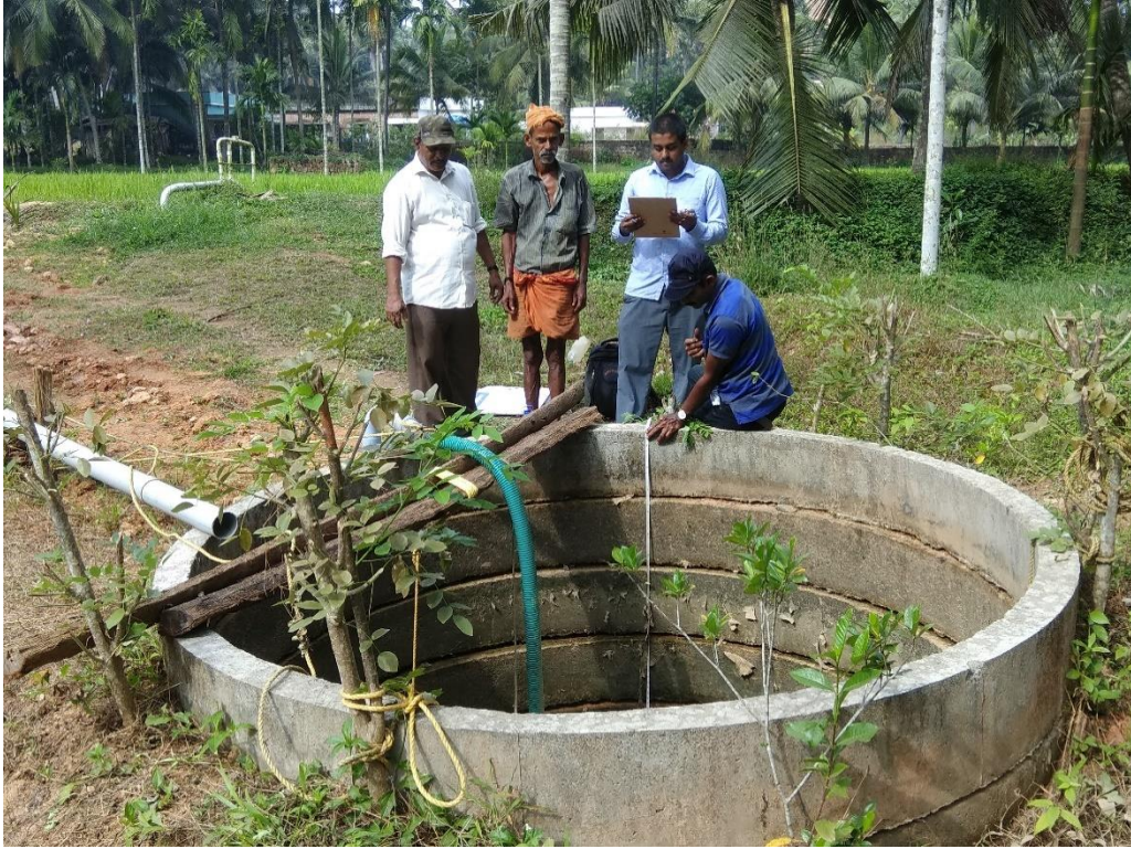
Fig. 3 Pumping well no 3
