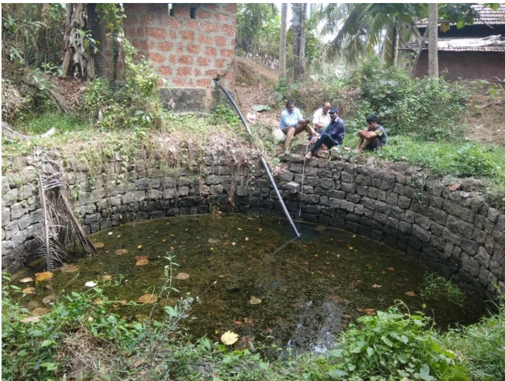
Fig. 2 Pumping well no 2
