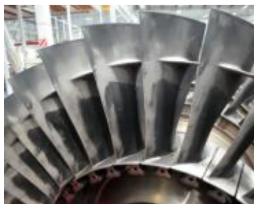
Figure 1.2 Corrosive deposits on compressor blade (Aust and Pons, 2019)
