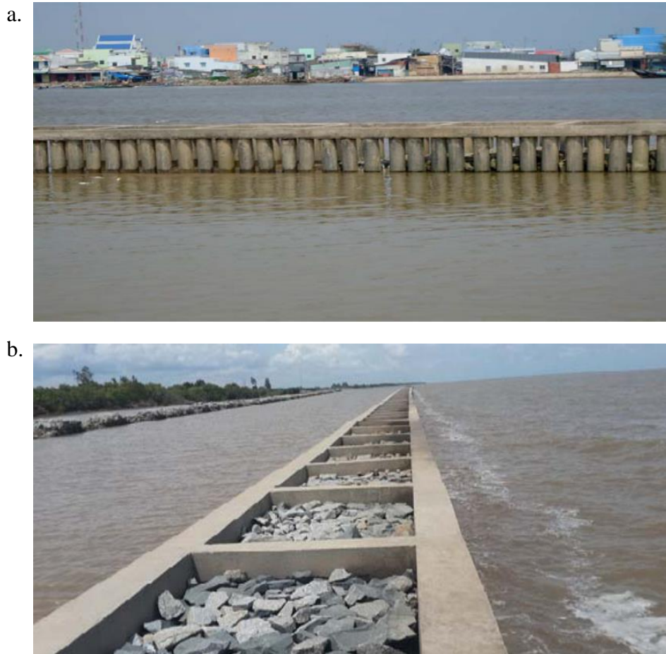
Figure 1.5 Double-row pile structure with rock core constructed at Dongying City, China (Xuan et al. 2020)
