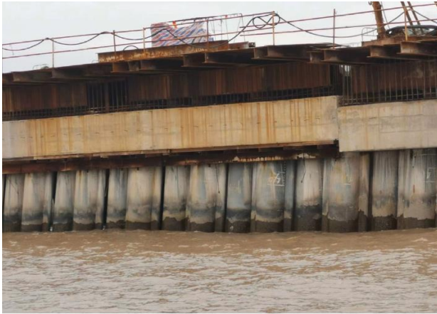
Figure 1.3 Pile breakwater under construction in Zhoushan Islands, East China (Yin et al. 2021)
